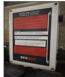
Push Button Controls
